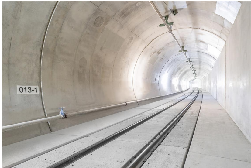
Caption 1: RAILONE safety system ROSS installed at Stuttgart 21 project (Picture: PCM RAILONE AG/ R. Mederer)
